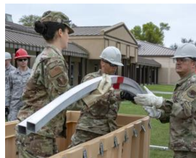
Members of Florida's Air National Guard practice building an Alaskan small shelter system at Jacksonville Air National Guard Base, Fla., Feb. 20, 2020. These heavy-duty tents can be equipped with electricity and climate control for use in deployed locations around the world. Photo By: Air Force Airman 1st Class Jacob Hancock. https://www.defense.gov/observe/photo-gallery/igphoto/2002256772/
