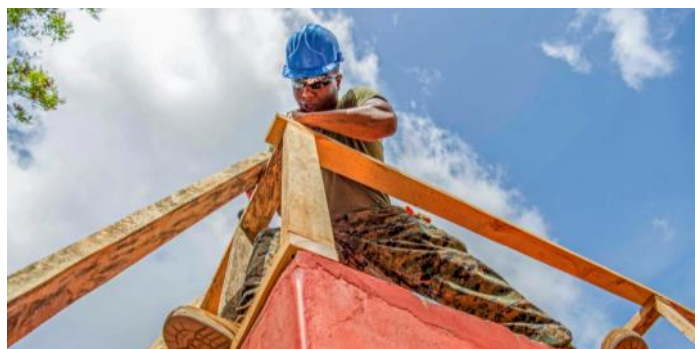
Marine Corps Sgt. Nicholas Harris joins lumber while building a school roof during Pacific Angel 18-4 in Vavuniya, Sri Lanka, Aug. 14, 2018.
